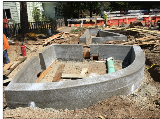
Stormwater Planter on Jefferson St.
