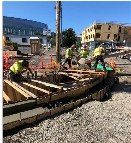
Stormwater Planter on Garden Avenue
