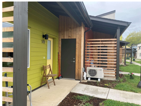
Electric heat pumps at Peace Village, a multi-family housing site in Santa Clara.
