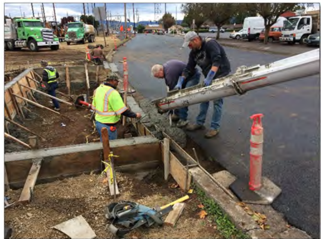
Stormwater Planter on Jacobs Drive
