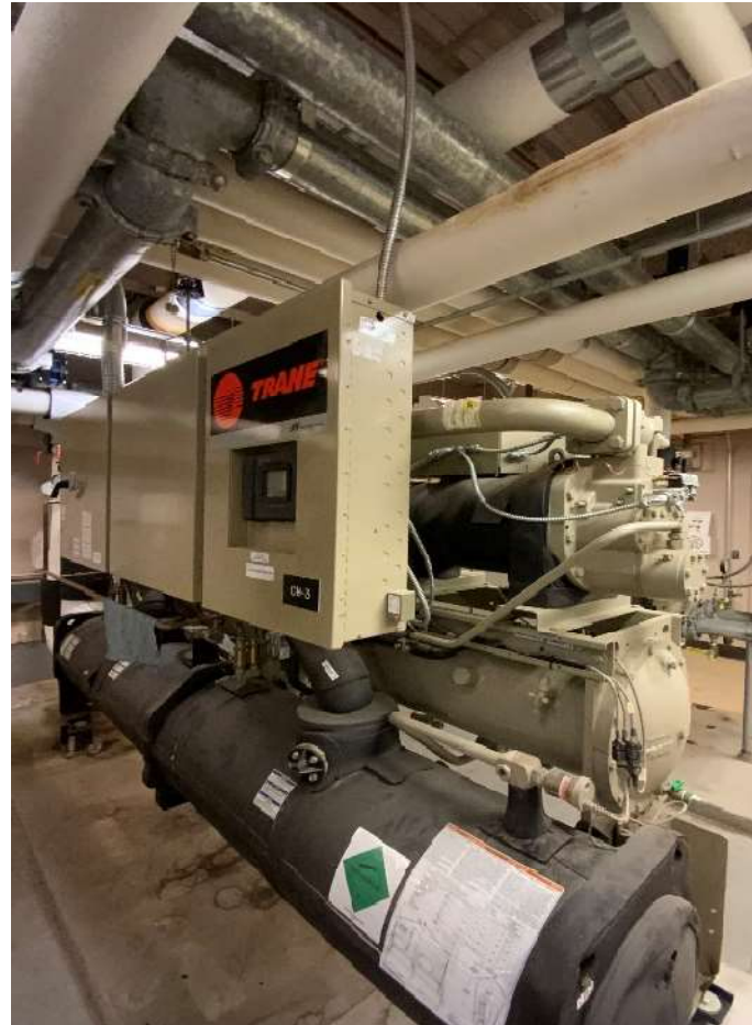
FIGURE 4-18 NEW CHILLER #3 OF 2016 TERMINAL UPGRADE
