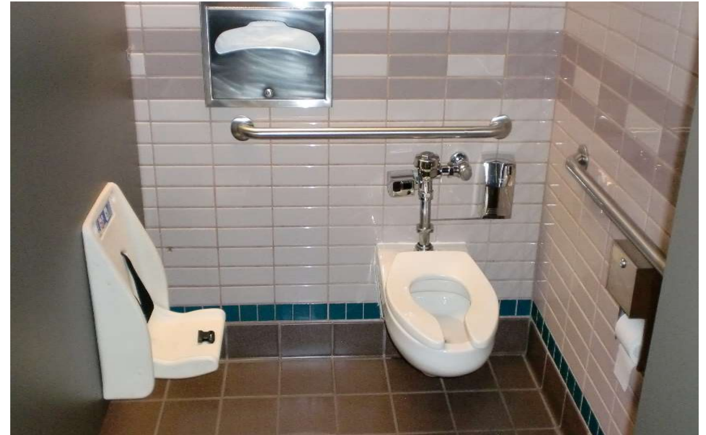
FIGURE 4-28 EXISTING WC AT LANESIDE RESTROOM
