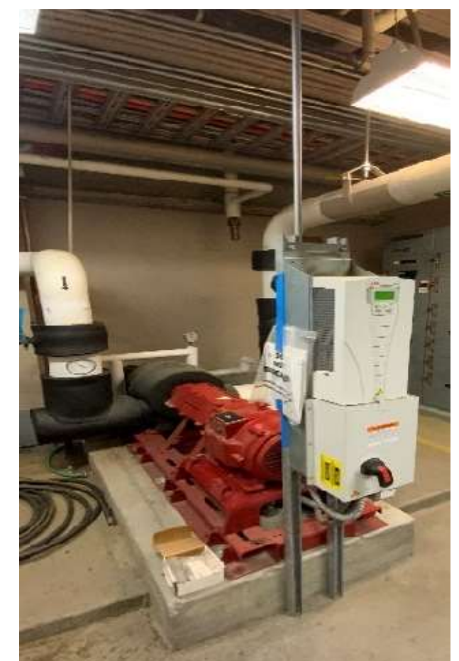
FIGURE 4-21 LEAD CHILLED WATER SECONDARY PUMP WITH VFD
