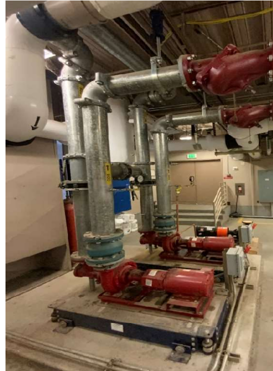
FIGURE 4-22 CONDENSER WATER PUMPS AT BOILER ROOM
