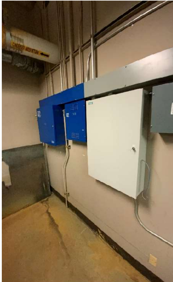
FIGURE 4-16 SIEMENS BAS CONTROL PANELS
