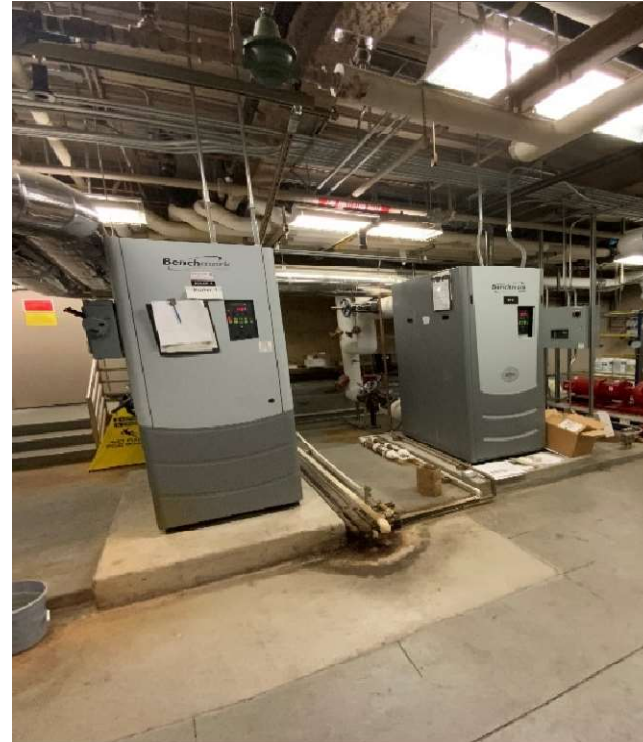
FIGURE 4-23 CONDENSING BOILERS IN THE BOILER ROOM
