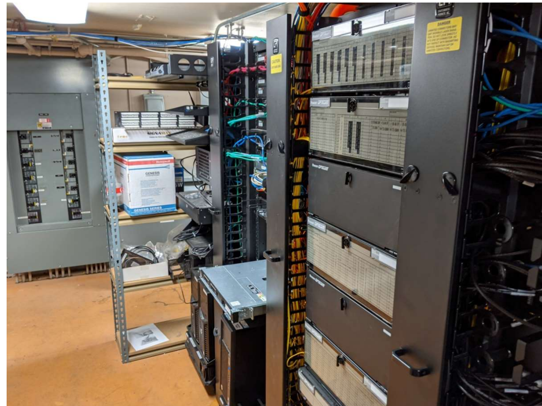
FIGURE 4-25 COMM ROOM ABOVE BAGGAGE HANDLING
