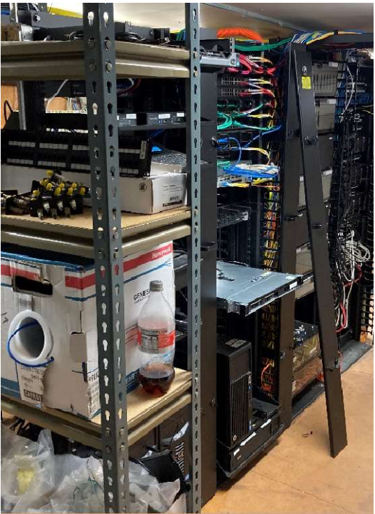
FIGURE 12-11 EXISTING EQUIPMENT RACKS IN MDF
