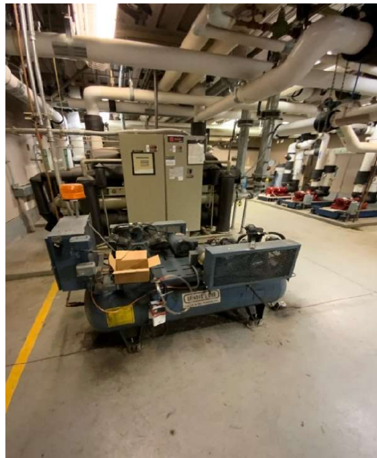
FIGURE 4-17 AIR COMPRESSOR SERVING EXISTING PNEUMATIC CONTROLS
