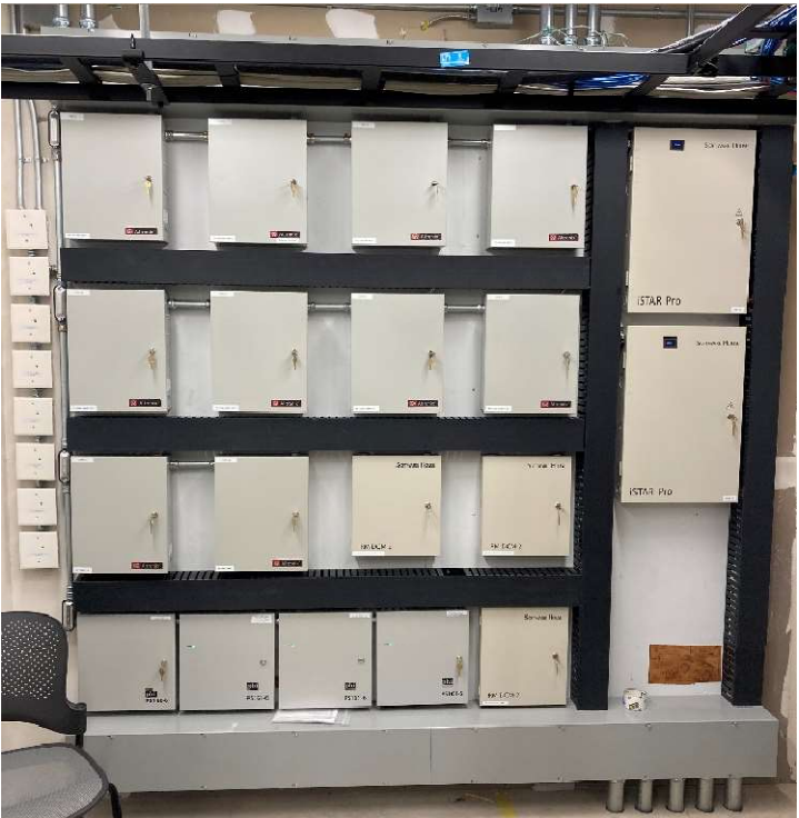
FIGURE 12-10 EXISTING WALL-MOUNTED SECURITY EQUIPMENT IN MDF
