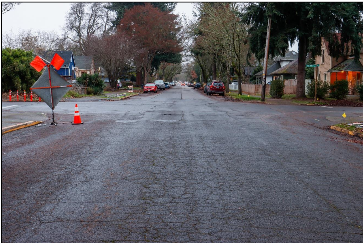
Existing Pavement Condition on W 8th Avenue
