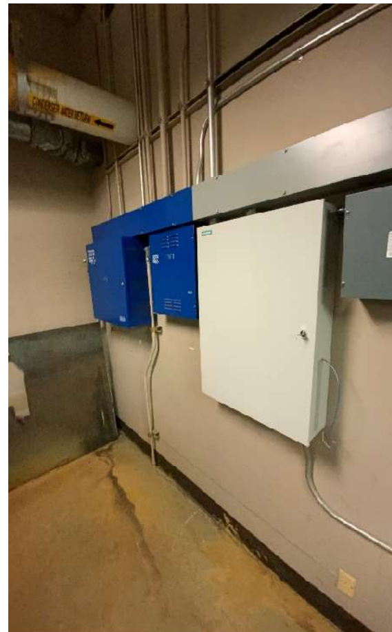
FIGURE 4-16 SIEMENS BAS CONTROL PANELS
