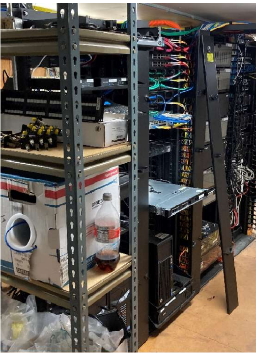
FIGURE 12-11 EXISTING EQUIPMENT RACKS IN MDF
