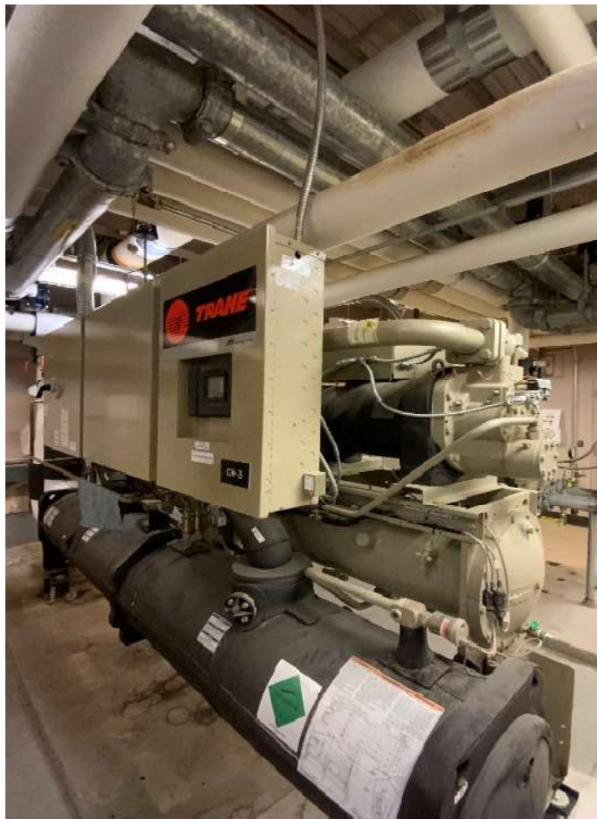
FIGURE 4-18 NEW CHILLER #3 OF 2016 TERMINAL UPGRADE
