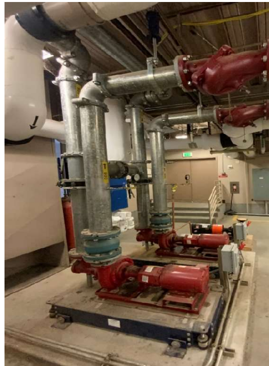
FIGURE 4-22 CONDENSER WATER PUMPS AT BOILER ROOM
