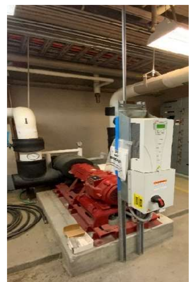
FIGURE 4-21 LEAD CHILLED WATER SECONDARY PUMP WITH VFD
