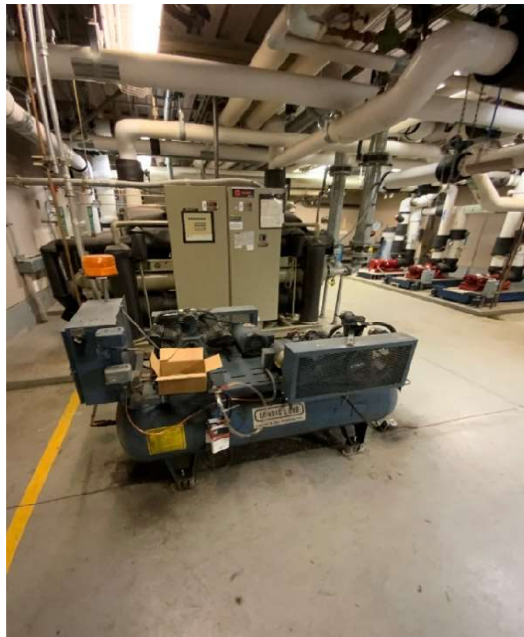
FIGURE 4-17 AIR COMPRESSOR SERVING EXISTING PNEUMATIC CONTROLS
