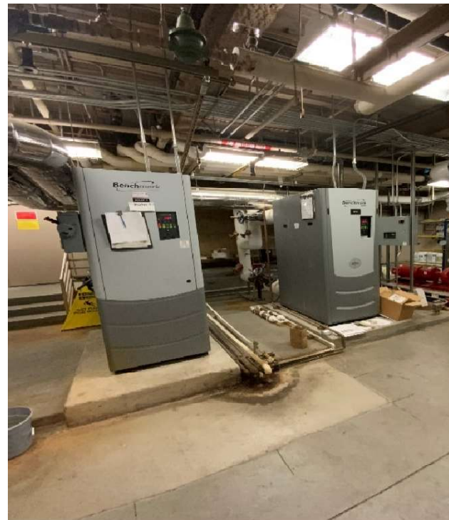
FIGURE 4-23 CONDENSING BOILERS IN THE BOILER ROOM
