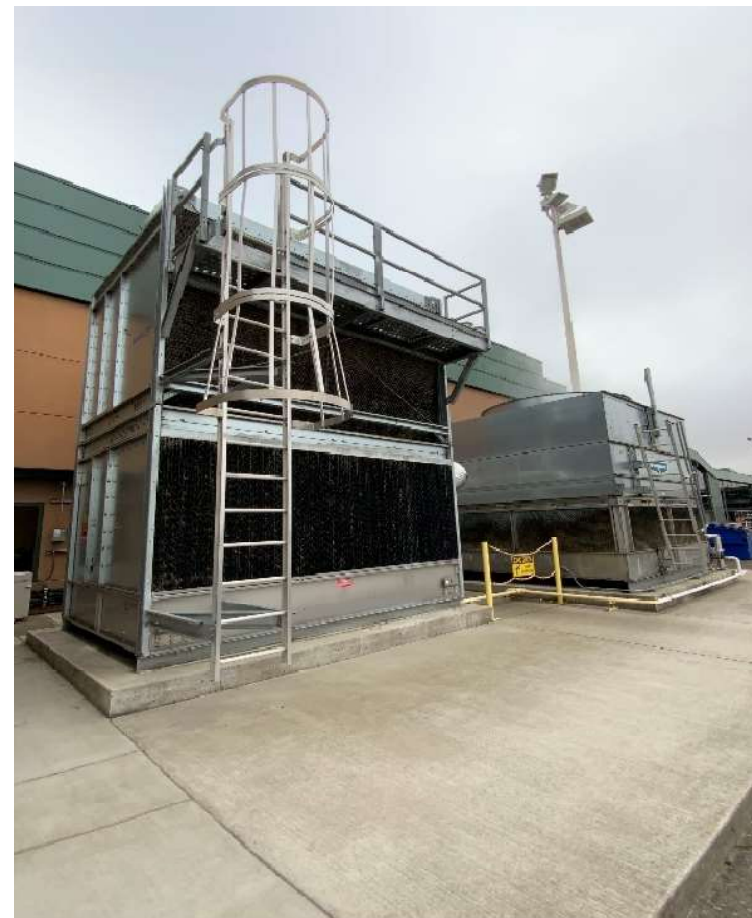
FIGURE 4-20 FLUID COOLERS AT CONCOURSE A
